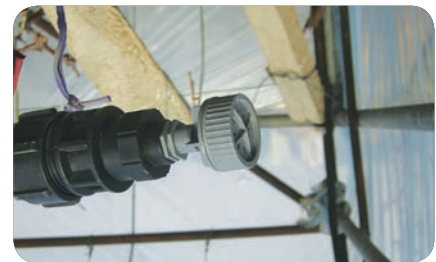
Application for sprinkler, fogger etc
